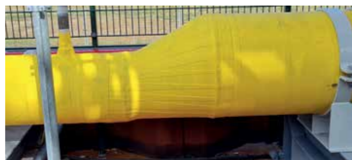
Coatings are moving beyond mitigating the effects of corrosion to actually stopping it from occurring
